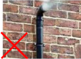
Surface mounted services
