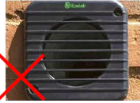
Surface mounted services
