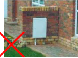
Visible service boxes
