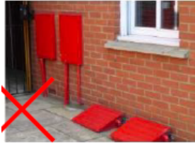
Visible service boxes
